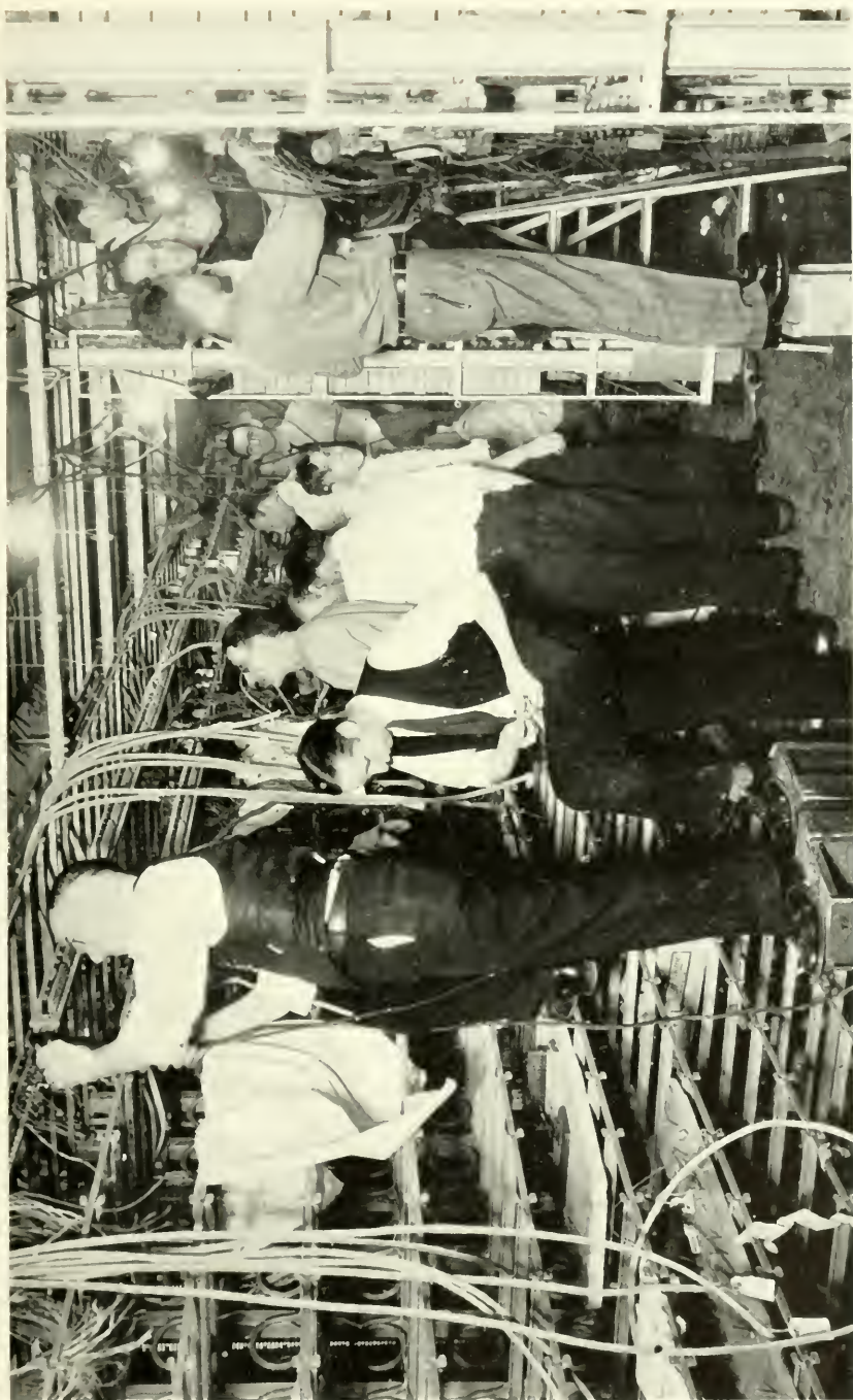
FIGURE 5. SOME OF THE 100 WESTERN ELECTRIC INSTALLERS WORKING ON THE HORIZONTAL SIDL OF THE INTERMEDIATE DISTRIBUTING FRAME AND RELAY RACKS.
